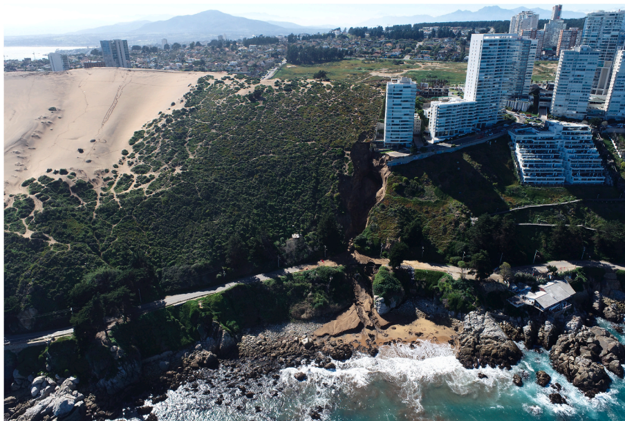
Fig. 1. The Kandinsky Building, a 17-story structure, experienced critical structural instability due to retaining wall failure and extreme precipitation events, intensified by the El Niño Southern Oscillation (ENSO). The incident led to mandatory evacuation and highlighted the vulnerabilities of coastal infrastructure, particularly when constructed on coastal systems, in the context of changing climate conditions. Nevertheless, the underlying cause of this catastrophe is intrinsically tied to extreme urbanization occurring on a dune system.
